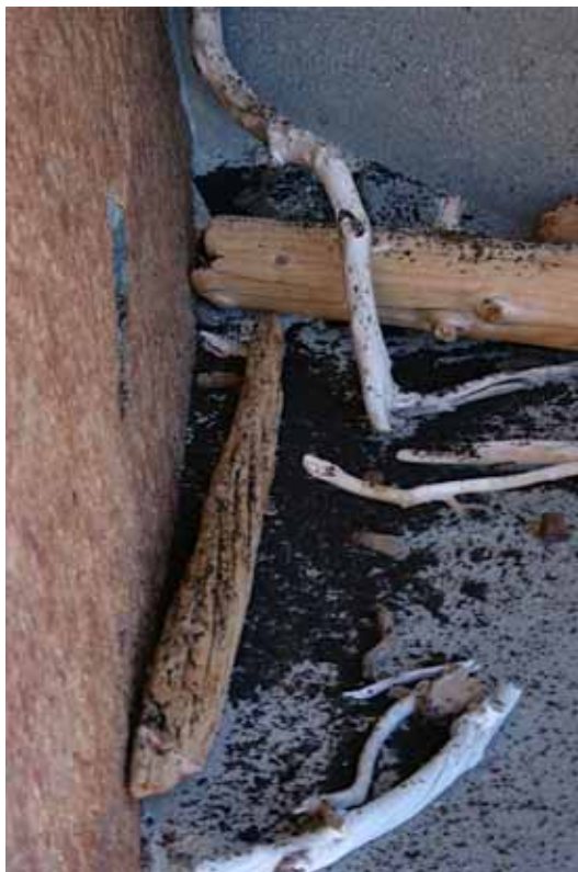
French Meadows Powerhouse - guano deposition indicating extensive night roosting activity by bats in alcoves
