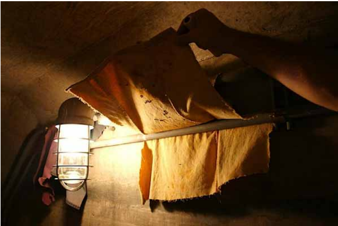
Ralston Afterbay Dam - guano on spare rags in galley
