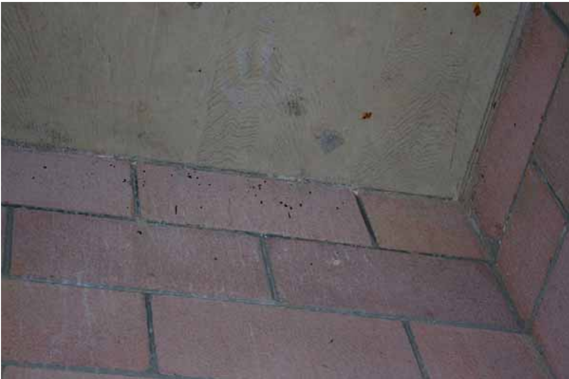
Hell Hole - Middle Fork Tunnel Gatehouse - minor night roost area inside gatehouse
