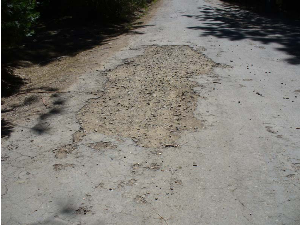
Photo R-2-3. Example of poor condition pavement along Middle Meadows Campground Access Road (14N28). (8/2108)
