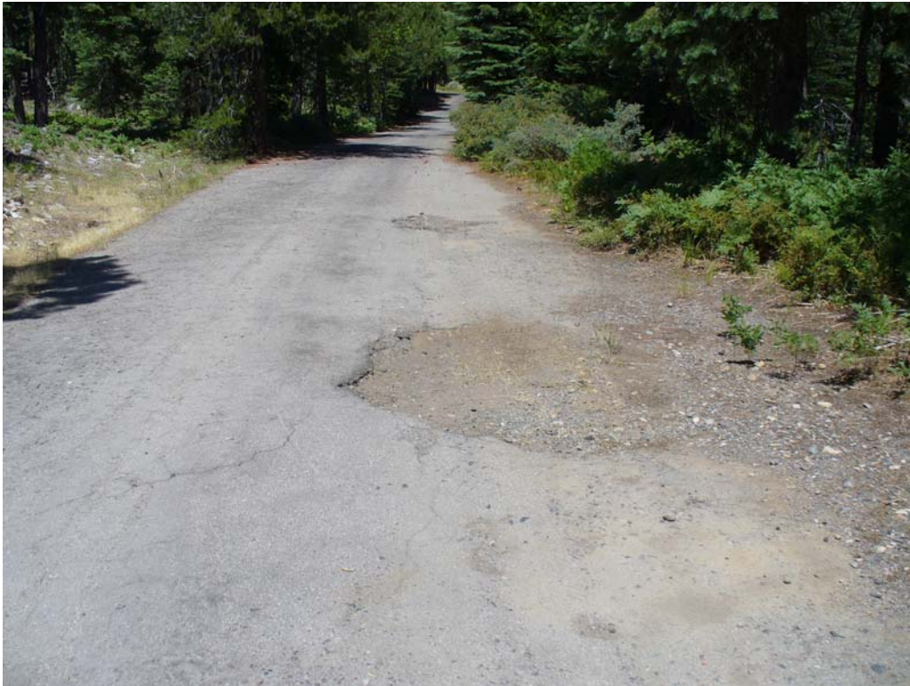
Photo Q-2-3. Potholes and damaged pavement along access road to McGuire Picnic Area, beach, and parking area. (7/24/08)
