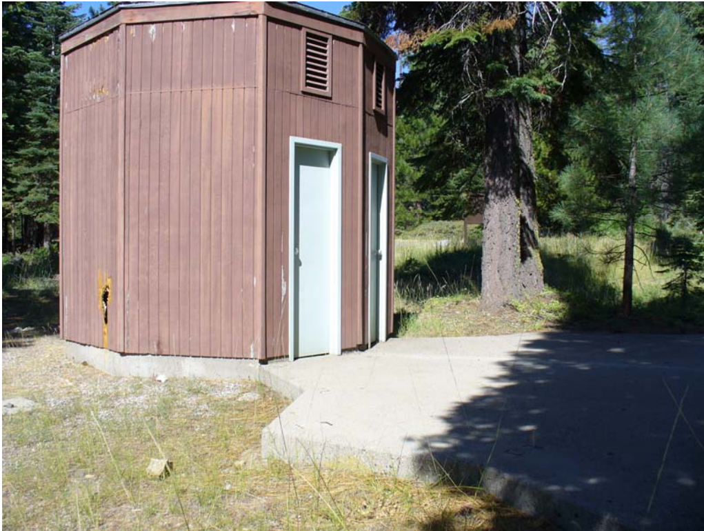
Photo Q-2-11. Backside of bathroom building. Space behind blue doors is now used for storage. Concrete pad was formerly a changing area. Note damage on building and large lip on concrete pad. (7/24/08)
