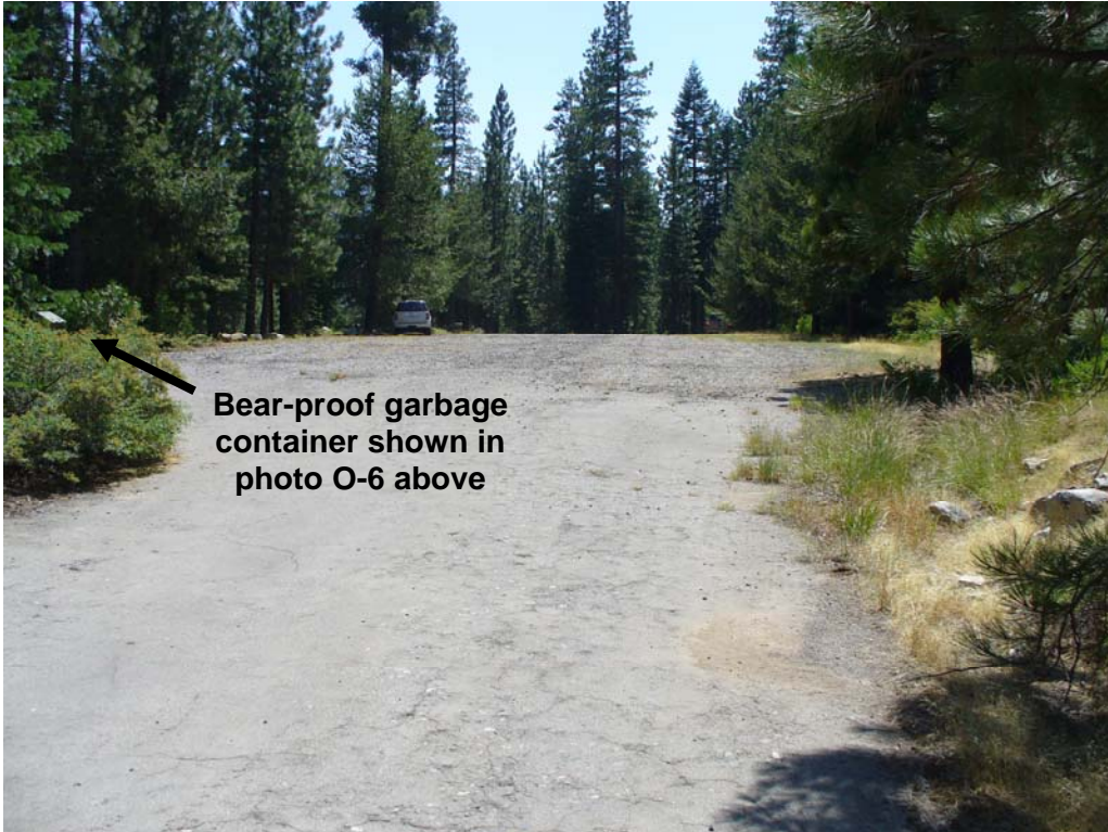
Photo Q-2-4. McGuire Picnic Area and Beach parking area. Note deteriorated asphalt surface. (7/24/08)
