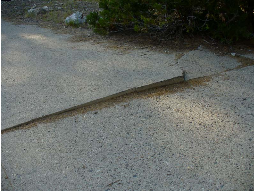
Photo P-2-4. Uplifted concrete at edge of high water turn-around area. (7/23/08)
