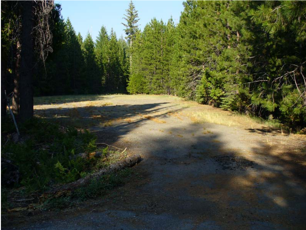
Photo P-2-9. South entrance to McGuire Boat Ramp Parking Area – northeast lot. Surface has deteriorated to base rock and is in poor condition. (7/23/08)
