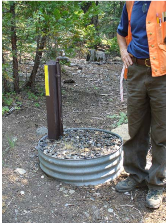
Photo O-2-19. Water faucet in picnic area. Does not meet accessibility standards due to handle design and level changes. (7/23/08)
