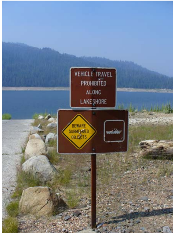
Photo O-2-3. Sign at upper end of French Meadows Boat Ramp. Sign is in good condition but paint is flaking. (7/23/08)
