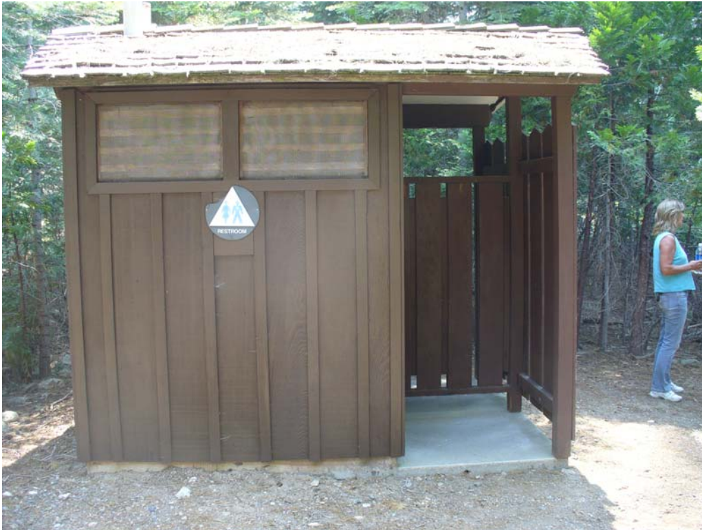
Photo O-2-17. Two-unit vault toilet located in French Meadows Picnic Area. This toilet does not meet accessibility standards due to narrow entrance width, level changes (e.g., concrete lip) and absence of hand rails. (7/23/08)
