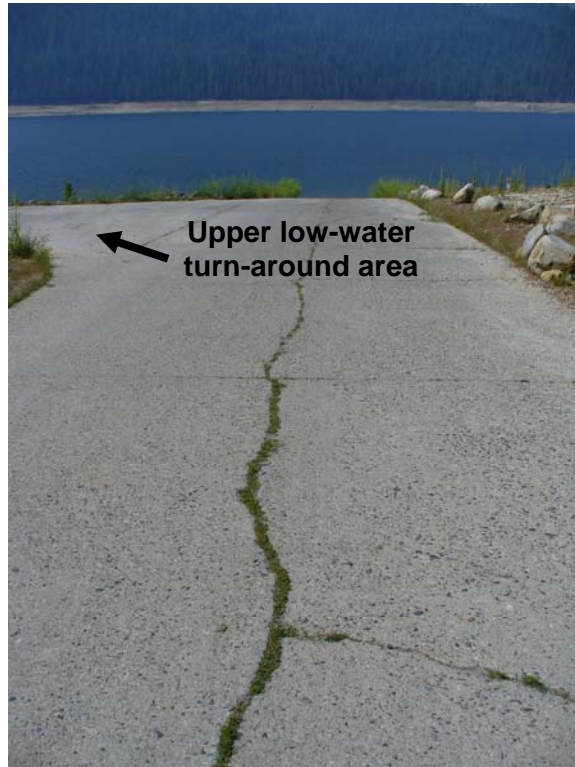
Photo O-2-2. Cracking in-filled with vegetation along French Meadows Boat Ramp, upper section. (7/23/08)
