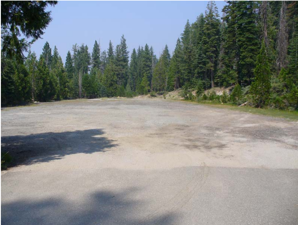
Photo O-2-5. French Meadows Boat Ramp Parking Area. Surface has deteriorated to aggregate base rock. (7/23/08)
