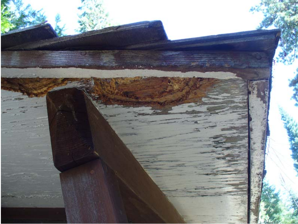
Photo K-2-11. Dry rot on bathroom structure No. 2. (9/04/08)
