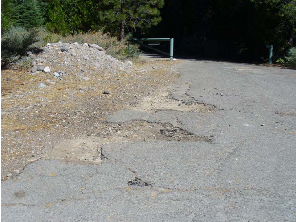
Photo D-2-4. Poor condition road surface at entrance to Big Meadows Campground. (8/21/08)
