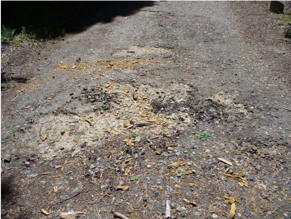
Photo D-2-9. Example of poor condition pavement in campsite spur. (8/21/08)
